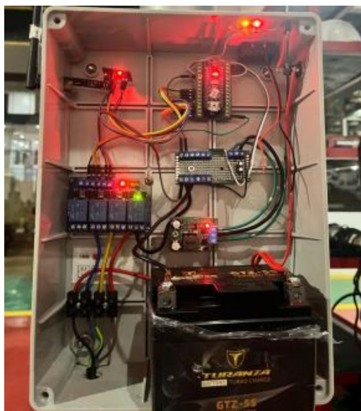
Figure 3. Electronic Installation Results
