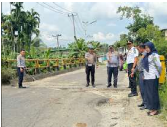
Figure 9. Road damage survey activities by students and the Transportation Agency and Police Agency
